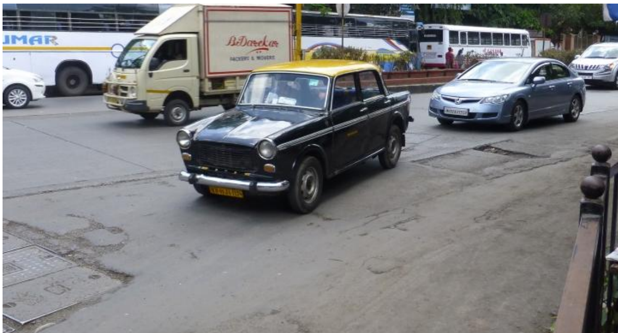
Figure 7: Pavement in poor condition
